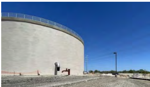
Location: San Antonio, TX Year Completed: 2023 Project: 2.0 MG Ground Storage Tank Owner: San Antonio Water System DN Tanks Scope: General Contractor Engineer: Tetra Tech, Inc.
