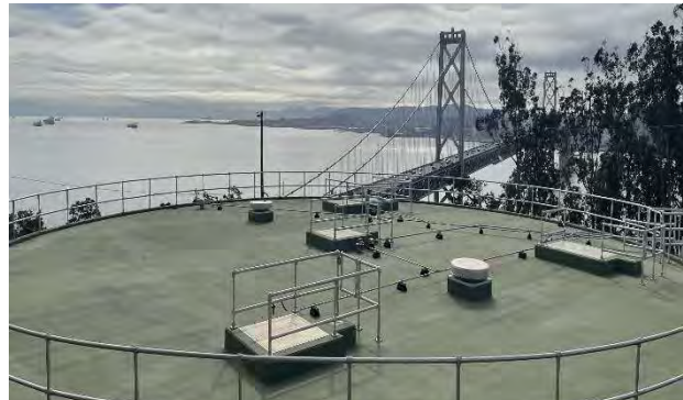
Tank Electrical/Instrumentation Conduits
