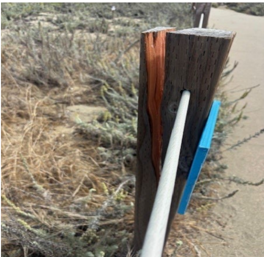
Damage to wooden post
