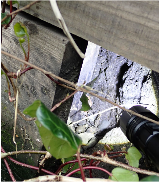
Figure 29 Soil loss behind upstream end of timber retaining wall at 2805 Naples Ave
