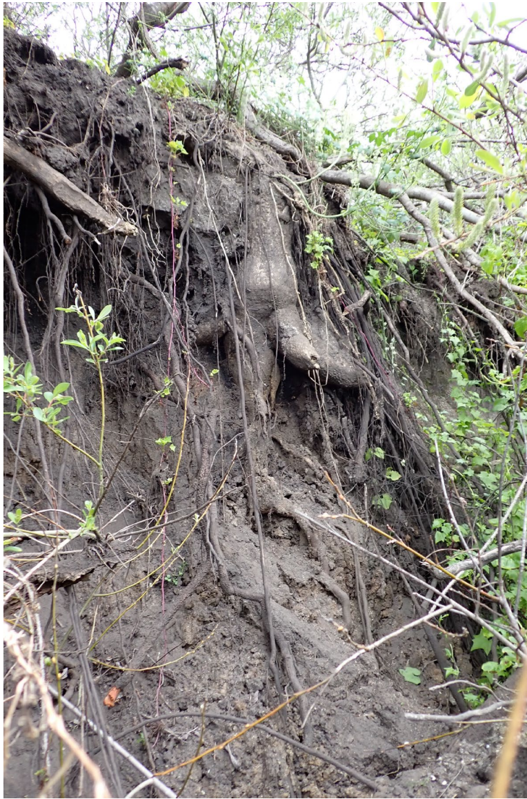
Figure 32 Example of undercut bank between Coastal Trail culvert outlets and Roosevelt Beach
