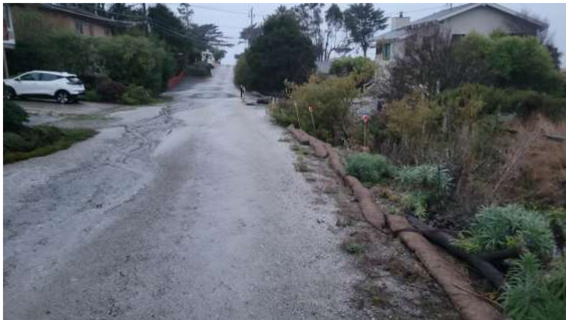
Photo 1. Rilling and creekbank erosion on 2nd Street. Channel incision and bank erosion have eroded the roadway embankment on north side of road. Lack of proper engineering of roadway causing rilling of roadway. View is looking west (downstream). Photo date: 11-22-2024.
