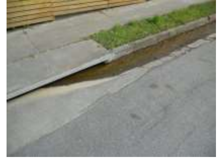
Photo 72 - Two Park stormwater drainage & runoff flows into pseudo storm drain at Santa Maria & The Alameda - then under The Alameda to an open-air ditch in its median
