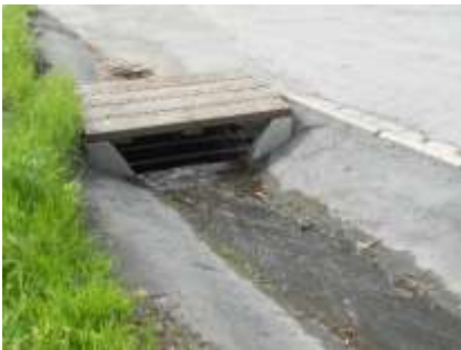
Photo 73 - Two Park stormwater drainage & runoff flows from the open-air ditch into a catch basin as entry into an underground storm system at The Alameda & Ave. Cabrillo
