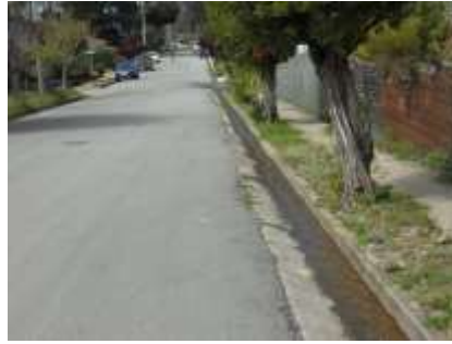
Photo 71 - Two Park stormwater drainage & runoff flows down Santa Maria from Columbus to The Alameda
