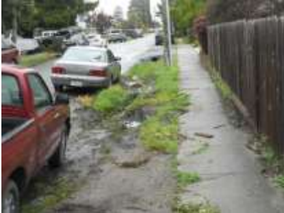
Photo 48 - Continuing runoff looking up San Carlos towards Francisco
