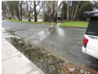
Photo 52 - Flooding over the eastern side of The Alameda to its median
