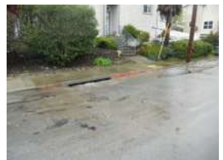
Photo 56 - Flooding down Ferdinand to underground storm system storm drain at Ave. Alhambra
