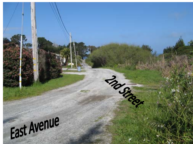
Photo 1 Photo taken from corner of 2 nd Street and East Avenue, looking west down 2 nd Street. A good-sized gully exists at photo left, between the telephone pole and pink flowering escallonia (see also Photo 3). The riparian area is in the photo on the right, on the other side of 2 nd Street and the dried Pampas grass. Note the large willow thicket in the middle of the photo.
