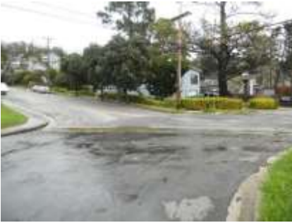
Photo 32 - Flooding down Ave. Portola to and over intersection with The Alameda
