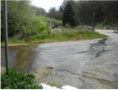
Photo 70 - Two stormwater drainage & runoff flows from Quarry Park entrance at Santa Maria & Columbus
