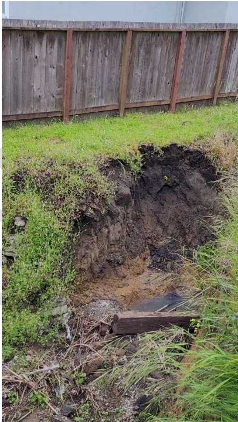
Figure 3 Gully on "East" between 4th and 3rd Sts.
