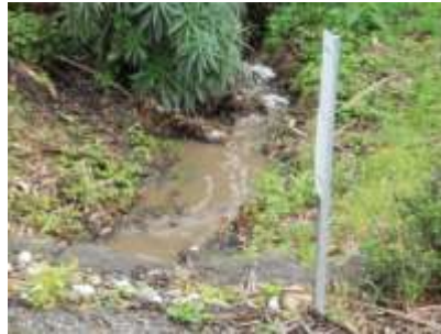
Photo 27 - Runoff from large pipe & culvert under Columbus at intersection with Ave. Portola
