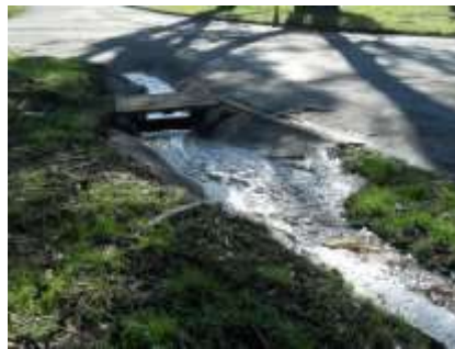
Photo 25 - Two stormwater drainage & runoff flows into underground storm system catch basin at The Alameda & Ave. Cabrillo from the open-air ditch
