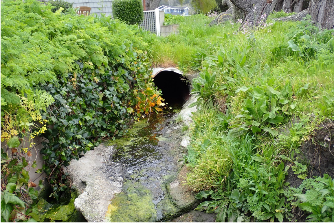
Figure 13 Outlet of 29" culvert under 2805 Naples Ave
