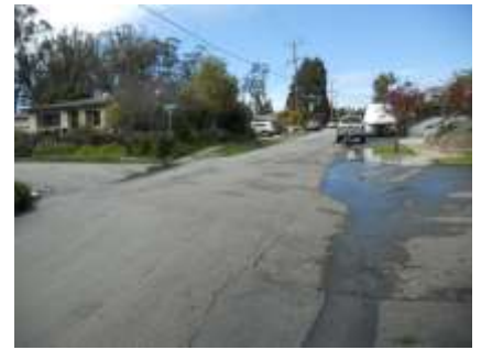
Photo 47 - Runoff down San Carlos and over x-street Francisco (looking up San Carlos)
