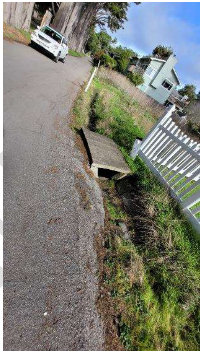
Figure 5 Overlarge Catch Basin Opening on Cypress
