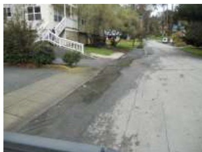
Photo 55 - Flooding down Ferdinand and over x-street Coronado (looking up Ferdinand)
