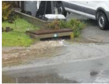
Photo 64 - Flooding from both sides into underground storm system storm drain at the westerly end of Sonora before where it curves toward Coral Reef
