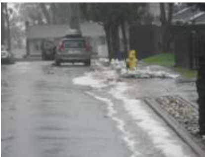
Photo 21 - Two stormwater drainage & runoff flows down Santa Maria over x-street Palma
