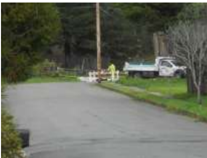
Photo 01 - Diverting lesser stormwater flow from Quarry Park at Park entrance (intersection of Santa Maria & Columbus)
