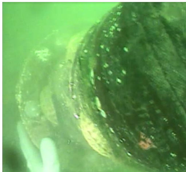
Exposed Flange of Riser
